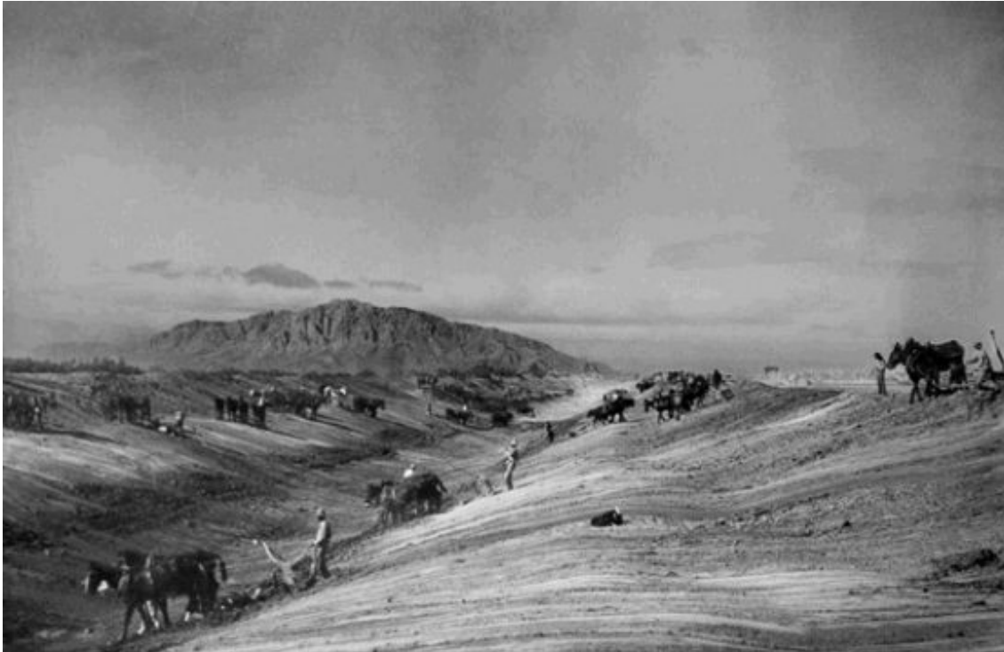
Early construction of the All American canal, with Mt. Signal in the background.
